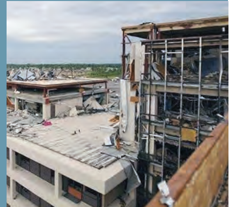
Figure 5: A photo taken from the roof of Mercy Hospital conveys the scope of the devastation. The hospital was a complete loss.
